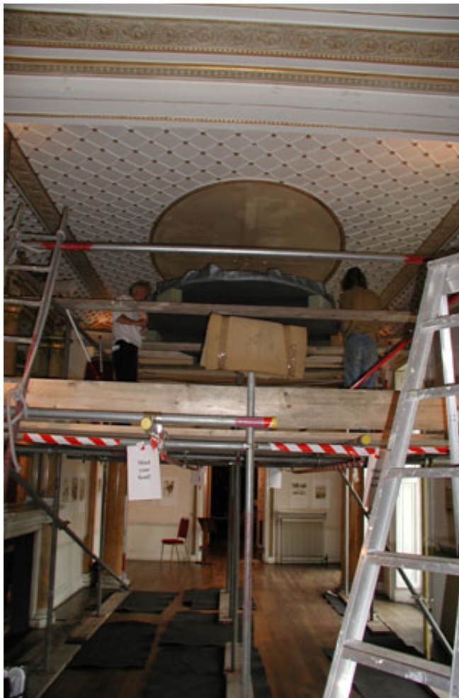
The Long Gallery filled with scaffolding as the oval oil painting is lifted back into place
